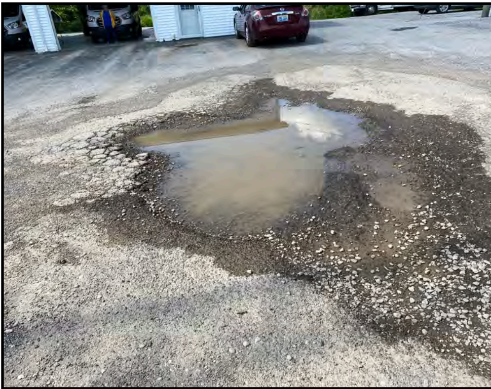
Photo 4. View of poor asphalt conditions.
